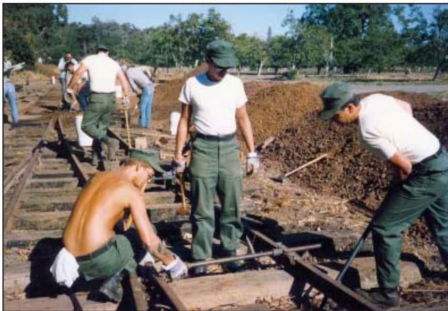
Navy Seabees check the gauge of the rails on the Deer Park passing siding Photo: Jack Burgess
