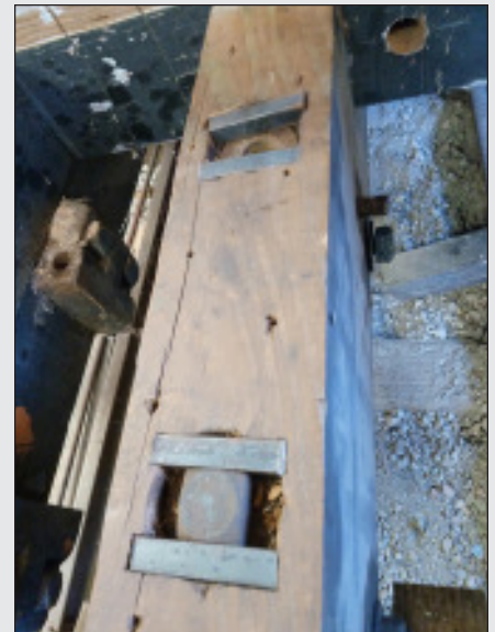
Draft timber showing non-traditional steel bar keyed insets to keep square head bolts from rotating. Draft post stops (cheek plates) visible on timber to left.
