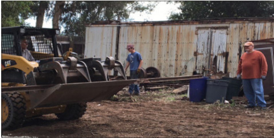
Brook Rother operated the Bobcat to move heavy rail, ties, wheel sets, and much more to clean up and organize the outdoor area in the corp yard, with the help of David Waterman (left) and Jay Shellen.
