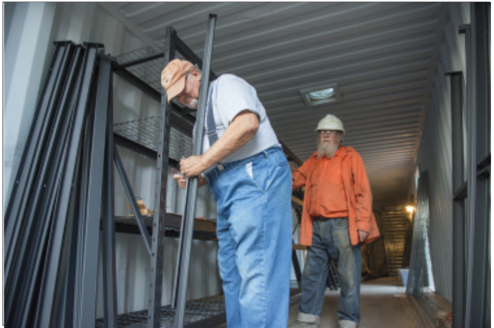
Jay Shellen (left) and Stuart Guedon (right) begin installing the shelving inside the new container - Bruce MacGregor photo
