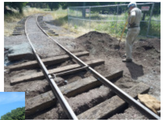
John Stutz replacing ties removed by EBRPD's contractor. Photo: Andrew J.L. Cary
