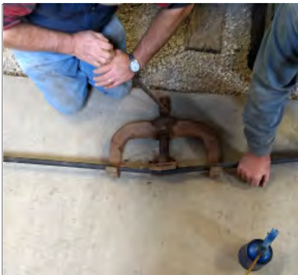
Bending truss rods with the 'armstrong' bender. A template is laid out on the concrete and the rod bent to fit the template. Andy is on the lever, Tony is holding the rod down.
