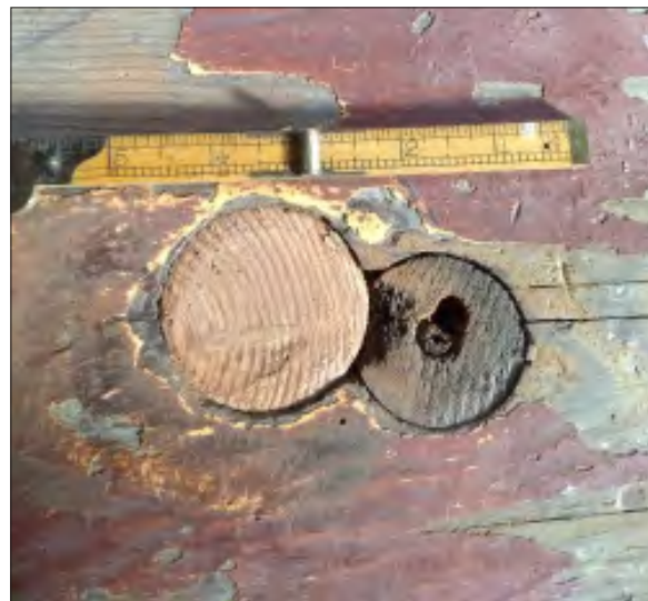
Plugging the buffer beam to allow a new brake staff hole to be drilled in a new position to match the one on the new railing. This obviously isn't the first time.
