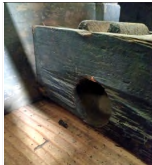
Inner body bolster buffer block showing body truss rod saddle directly above air pipe hole. New wood at bottom is the new bolster beam.
