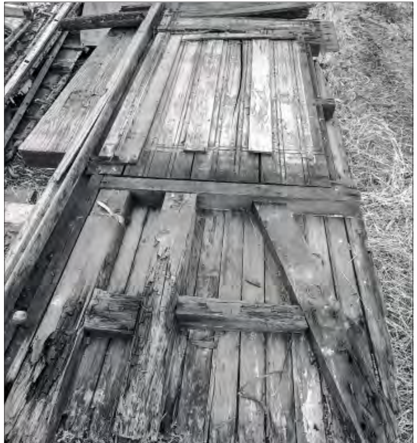
Figure 1. A circa 1990 interior view of roughly half an end wall, showing flood damage most dramatically visible close to the camera—on the parts of the wall closest to the end beam and car floor. This photo lines up with the right hand portion of John's 3D CAD reconstruction in Figure 2. Photo: Bruce MacGregor
