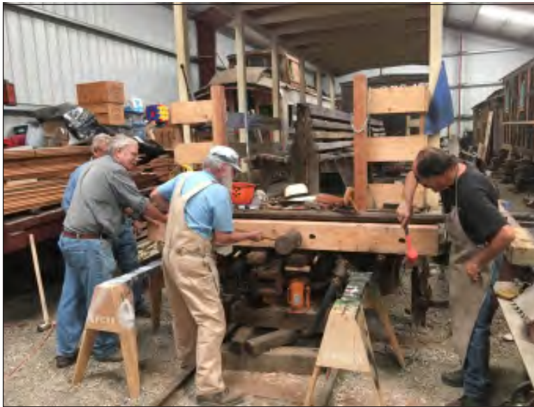
Restoration Crew fit new beam onto "A" end of flat car 1725. Photo: David Waterman
