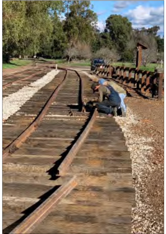
John Goldie and David Waterman (in coveralls) drill holes in joint bars to connect one of the last segments of track to the west Deer Park switch . Photo: JBurgess
