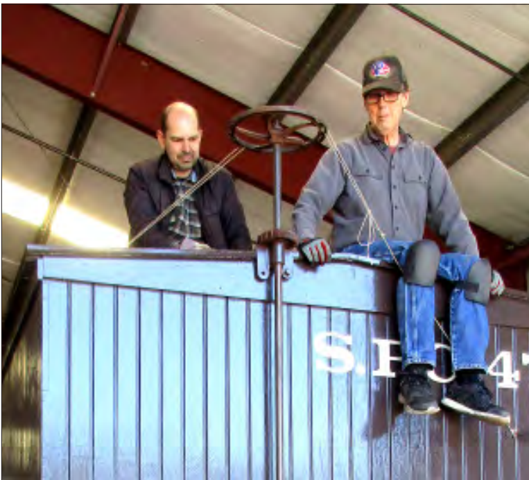
Josiah Larson (on left) with Tom Sturm working on the temporary roof of box car 472. Photo: Don Marenzi
