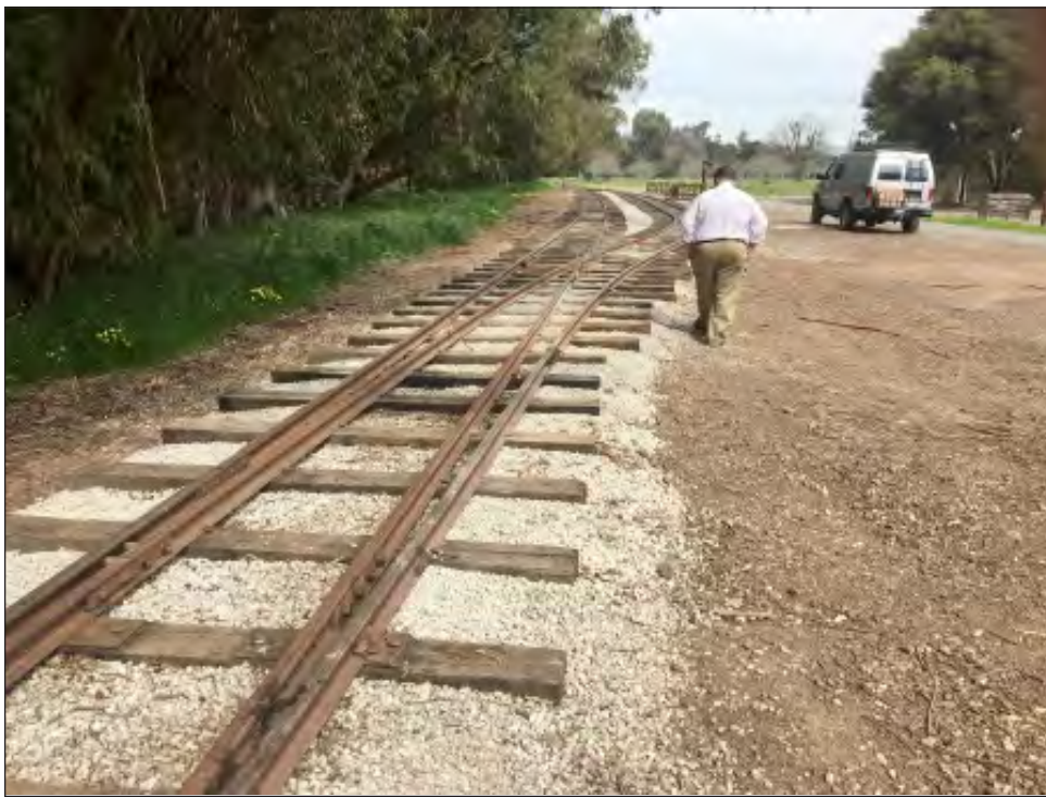
Registered Mechanical Engineer, David Mori, inspects final switch installation. Photo: Jack Burgess
