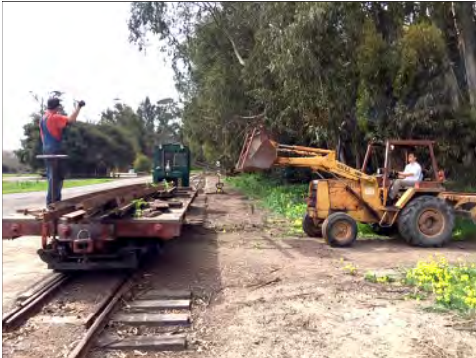
David Waterman (left) gives signal to Bobby Goldie (in tractor) as they cleanup track work debris. Photo: John Goldie
