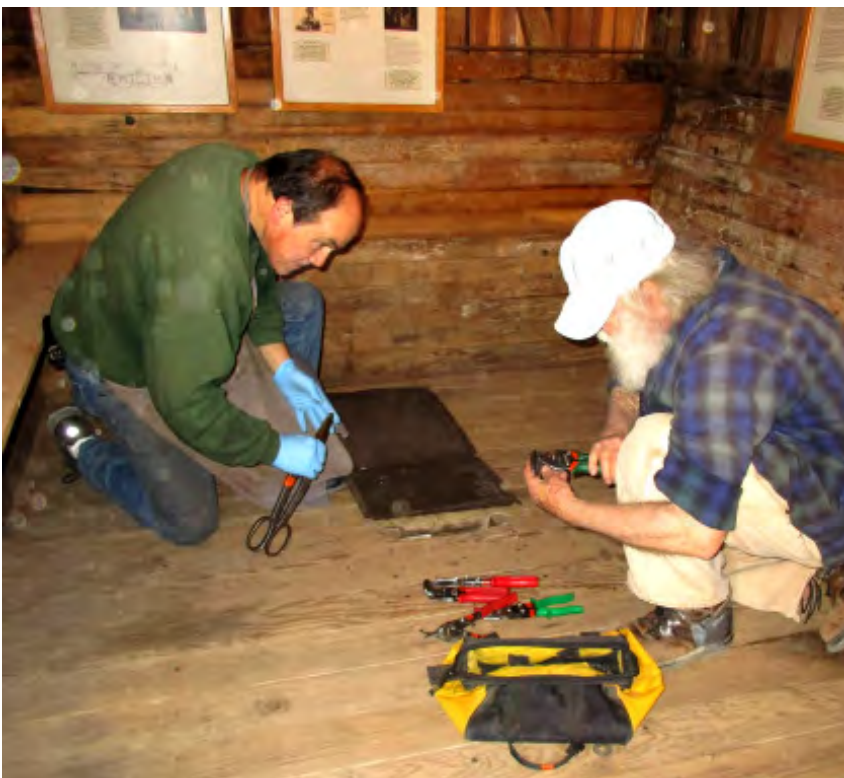
Ken Lippman (left) and Gene Arrillaga (right) made a metal cover to cover a hole in the floor of the museum car. This hole provides access to the center pin for the truck. Photo: Don Marenzi.
